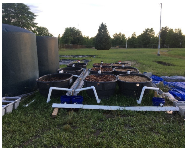
Building bioreactors as part of the study.
