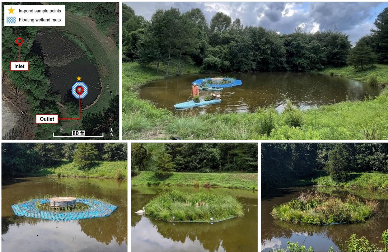
Armory Pond FTWs; top row: aerial imagery depicting FTW design and water quality sampling locations (left) and FTW installation (right); bottom row: FTWs directly following installation (left), approximately 12 months following installation (center), and approximately 24 months following installation (right).
