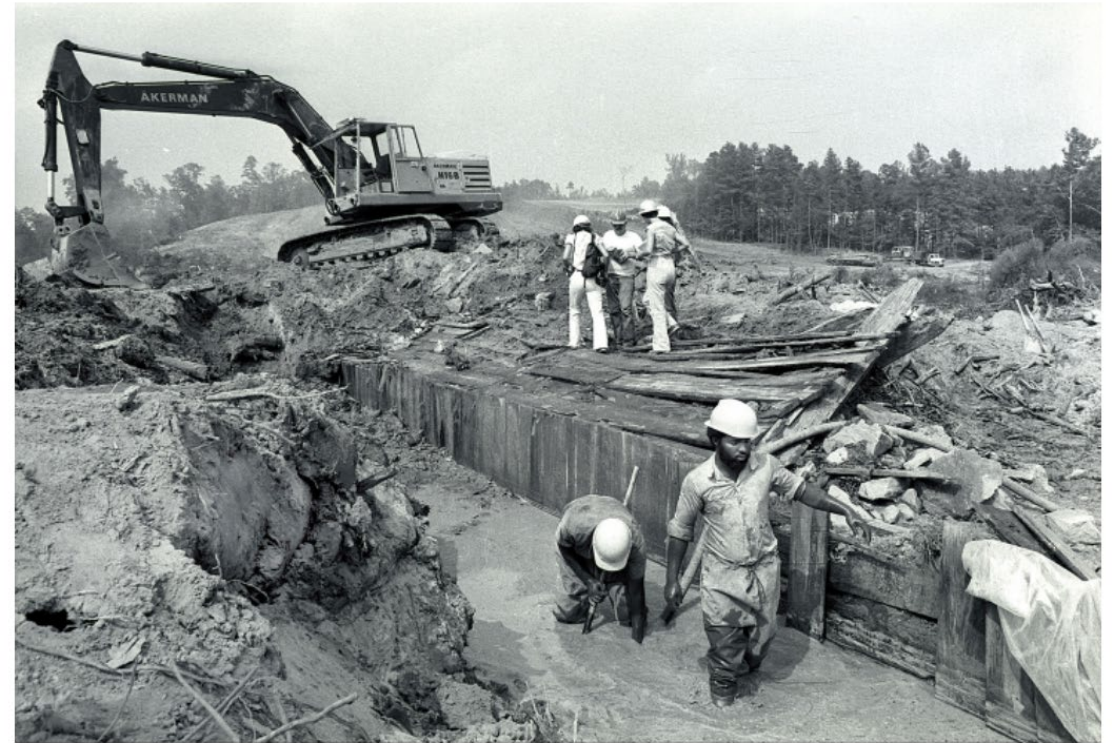
Photograph of workers on an old wooden dam uncovered during construction of Falls Lake Dam in the late-1970s. When this photo was taken, the wooden dam was over 150 years old and covered by silt, mud, and water. Photograph courtesy of the US Army Corps of Engineers.
